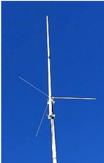
Typical vertical base station antenna
